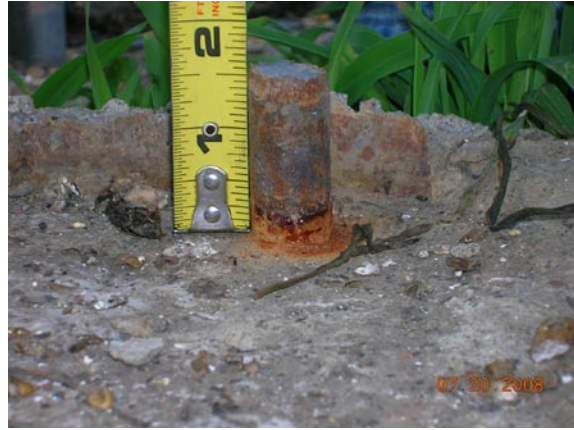
Failed anchor bolt.
