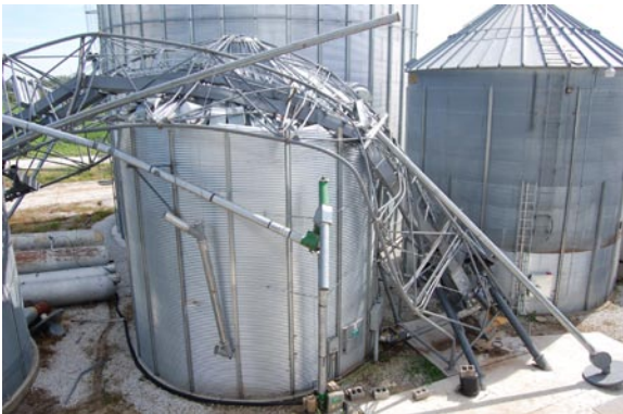
Base of collapsed tower.
