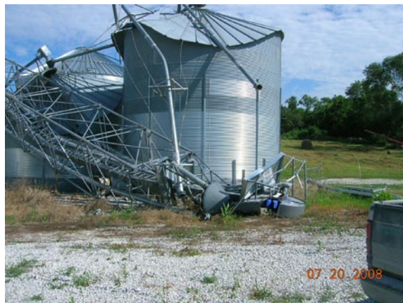
Top of collapsed tower.
