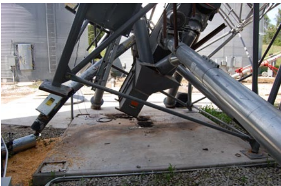
Foundation pad with two legs detached.
