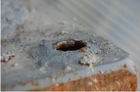
Failed anchor bolt weld.
