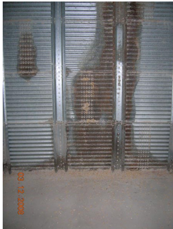
Rust near the base of interior.
