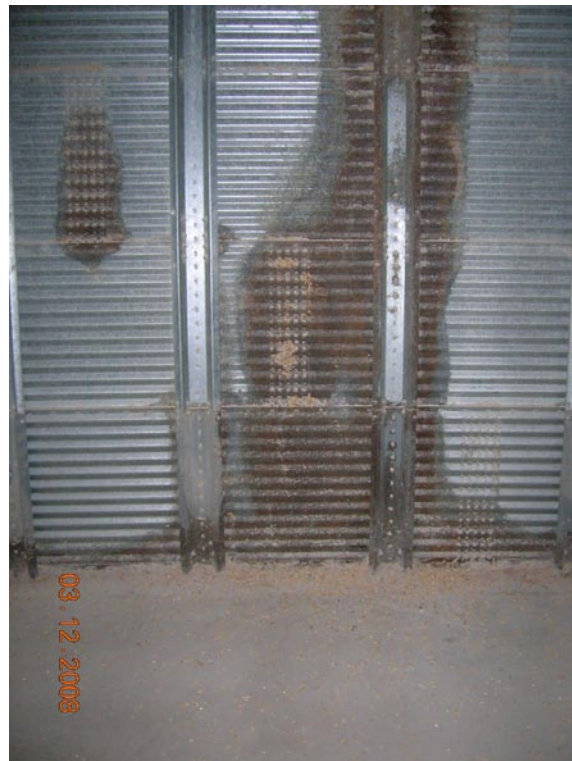
Rust near the base of interior.
