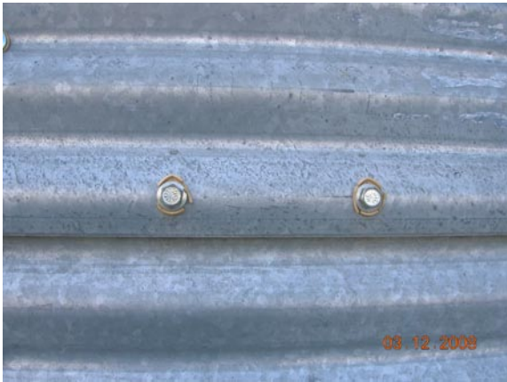
Damaged seal washers at horizontal seams.
