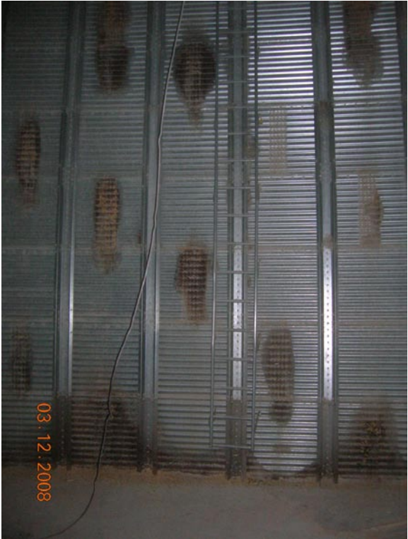
Rust at bolt locations.
