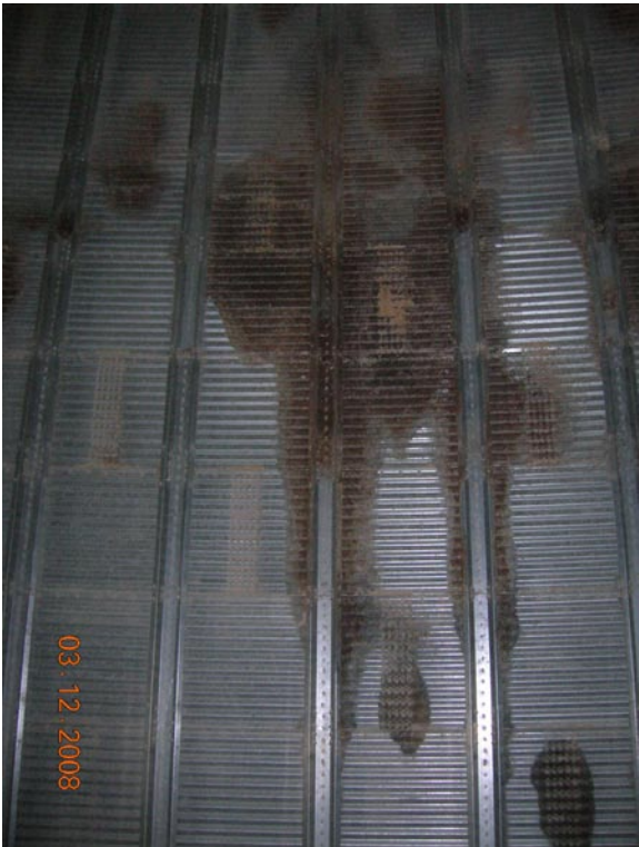
Severe rusting near some stiffeners.
