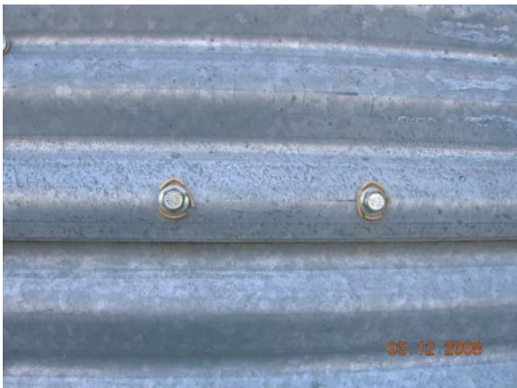
Damaged seal washers at horizontal seams.
