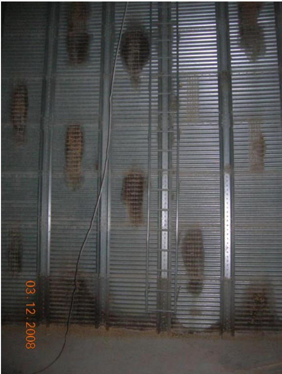
Rust at bolt locations.
