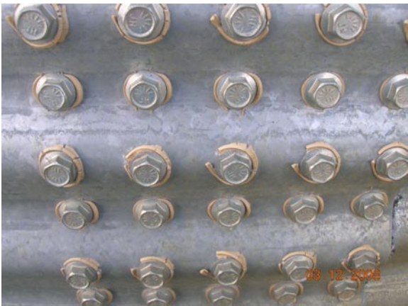
Damaged seal washers at vertical seams
