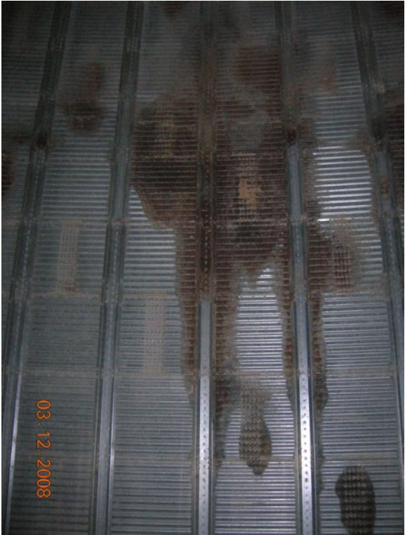
Severe rusting near some stiffeners.
