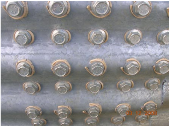
Damaged seal washers at vertical seams
